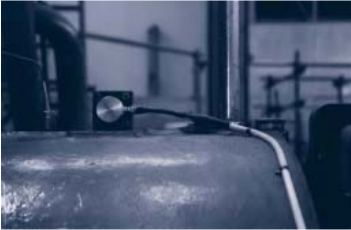
Pedestal vibration monitoring
