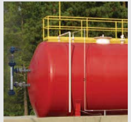
Fuel Oil Storage
